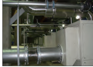
Suji WWTP (NX300), Korea
